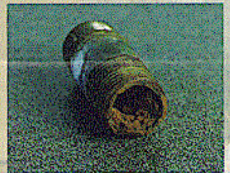
Here, one can see the effects of corrosion on extinguishment piping.
