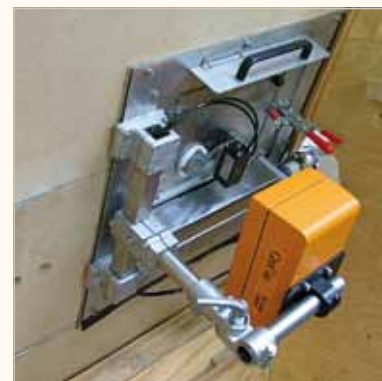
FMV in drop chute underneath dryer cyclone
